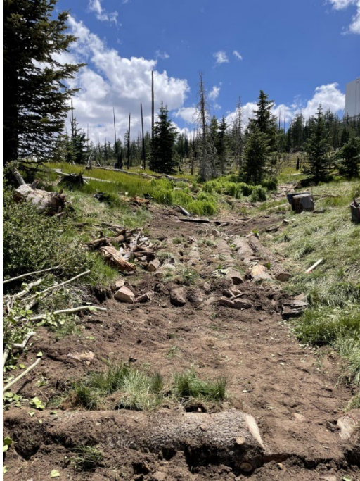
Figure 3. Log Mattress structure installed in Ash Creek to prevent further incision and catch sediment as part of the Highwater Cienega project.
