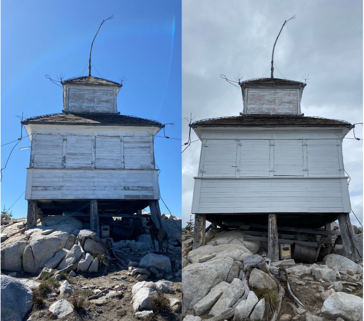
Figure 2. North 20 Mile D-6 Cupola (east side) before and after repairs and repainting
