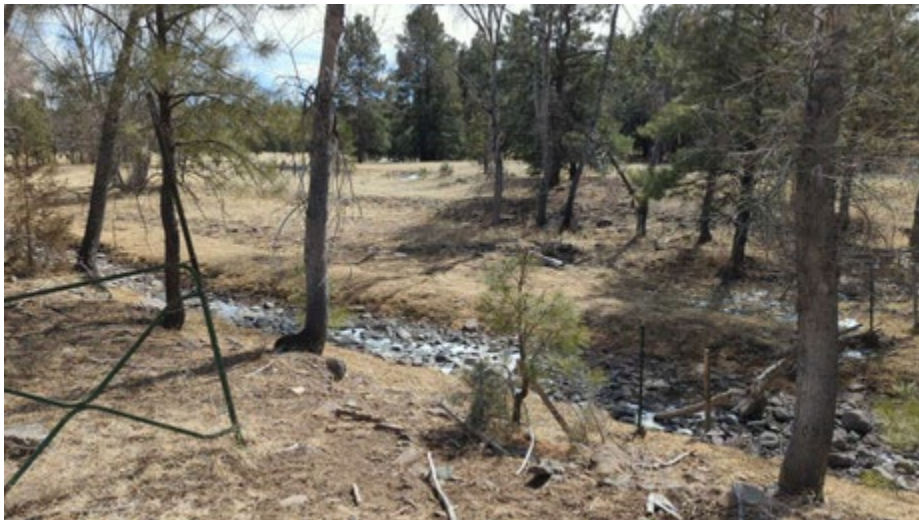
Gap in fence at FS / private boundary on downstream end. Photo looking towards private land.
