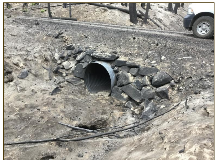
Figure 3 Engineers and hydrologists evaluate culverts like this one to evaluate its capacity to handle the predicted increased flows.
