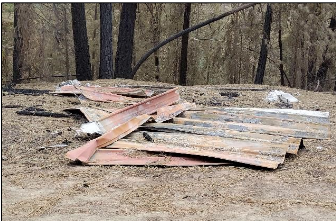
Figure 4 All that remains of the Wolf Creek TH toilet is the metal roof.
