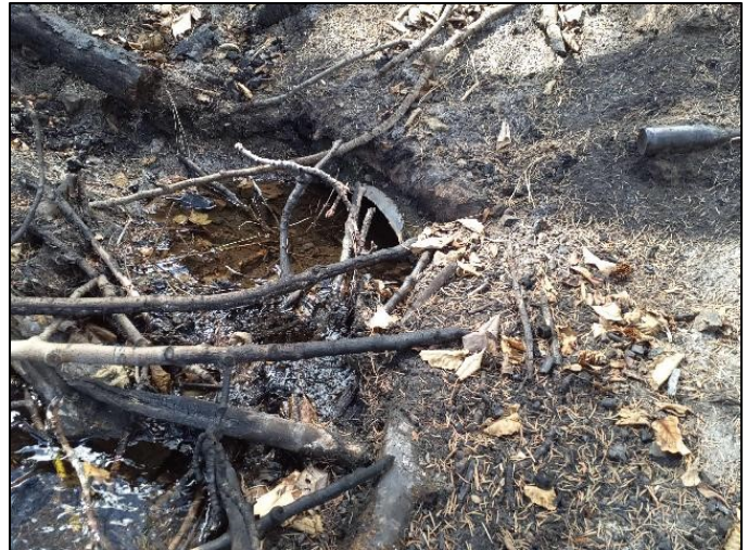
Figure 3 Burned debris can quickly plug undersized culverts.
