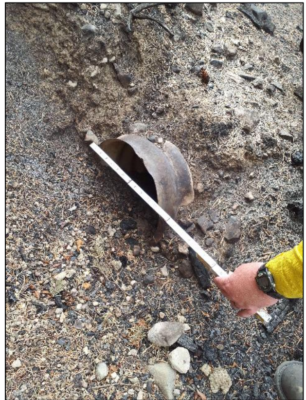
Figure 3 Plugged culverts can lead to a road being overtopped by flood waters.
