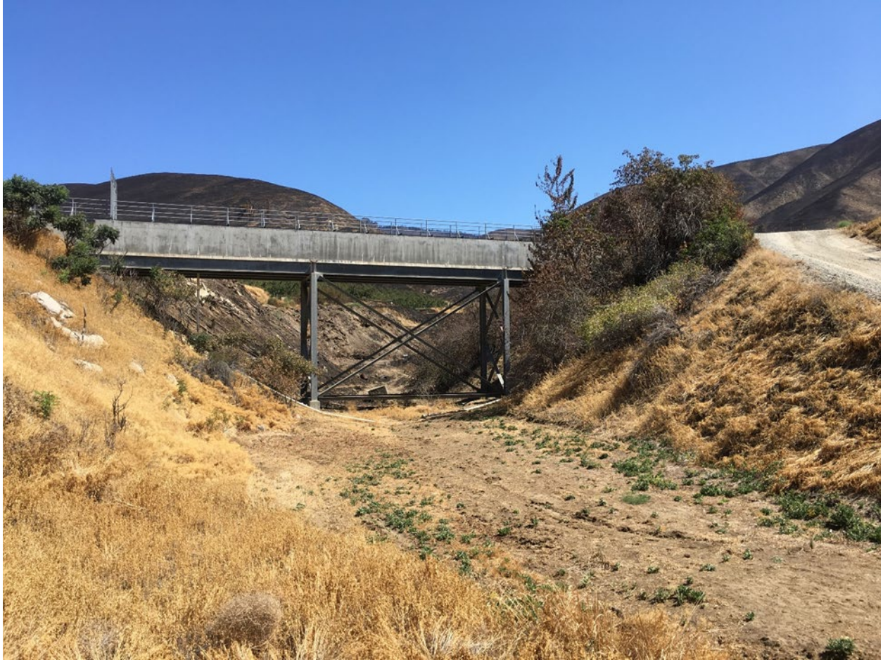
Figure 1. Photo taken where irrigation canal crosses unnamed drainage in a flume with high combined hazard for debris flows. This location is above the intersection of Kenoyer and Red Apple Roads (Location 4 on Plate 1).
