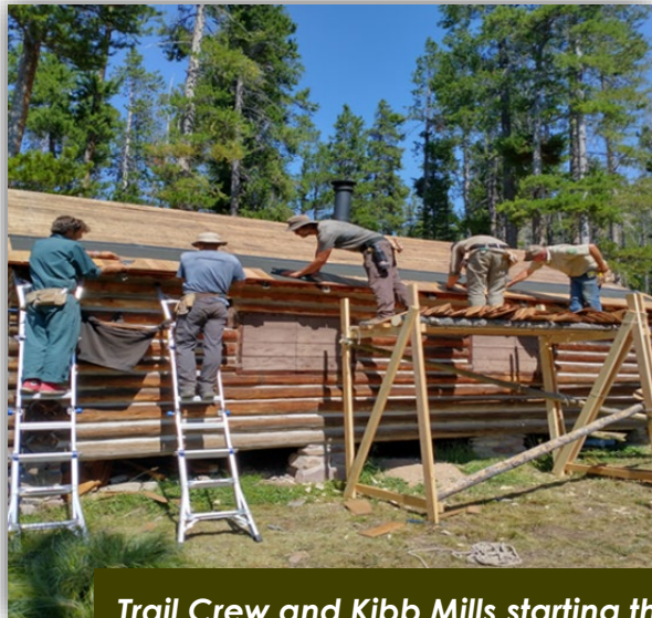
Trail Crew and Kibb Mills starting the first course of shingles on Carmichael Cabin
