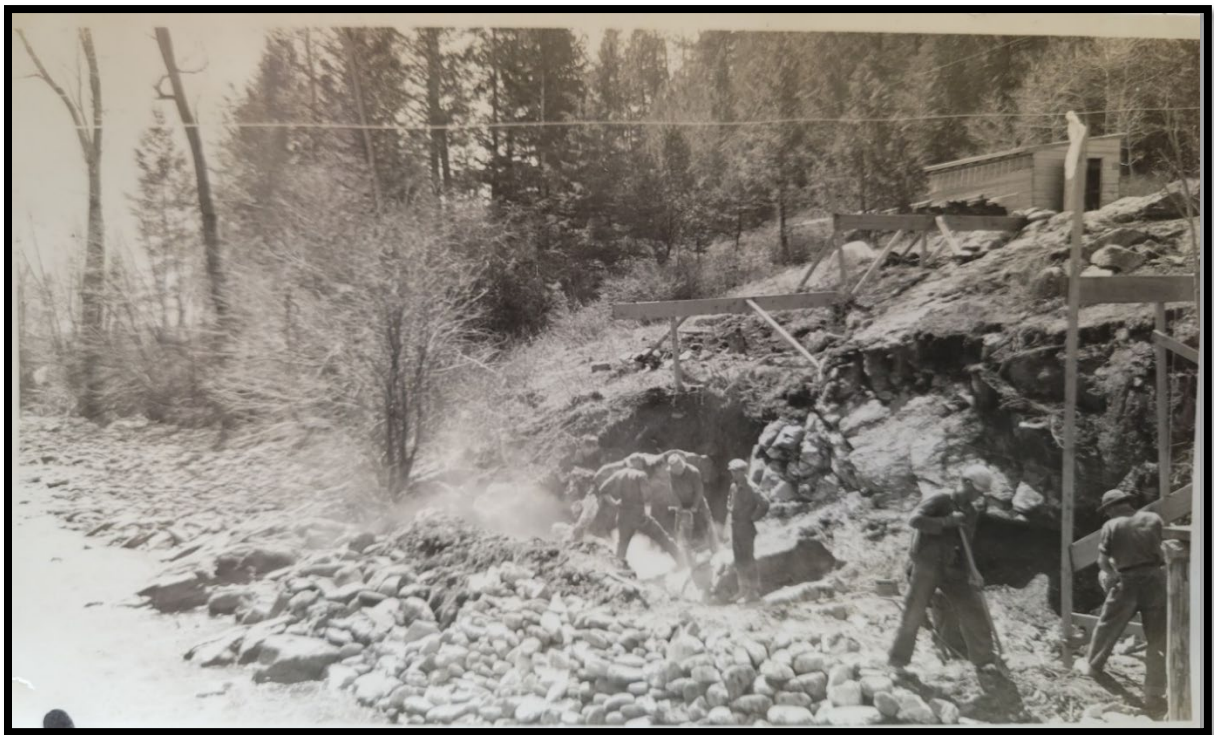
Figure 12. View of excavation for concrete footings with hand tools looking at west side of river April 26, 1935
