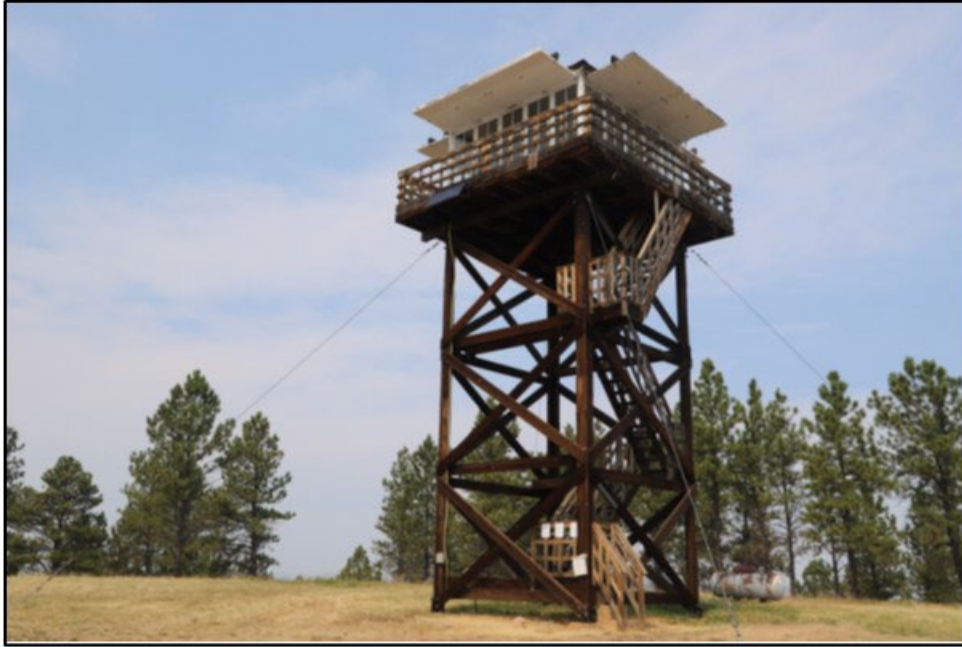
MT_RosebudCounty_PokerJimButteLookout_0002. Lookout, Site 24RB2233, Poker Jim Butte Fire Lookout August 26, 2021, View to Northwest (Urbaniak 2021)
