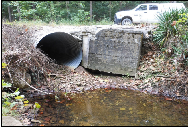
One of several culverts that impede passage of organisms and cause erosion that is proposed for replacement.
