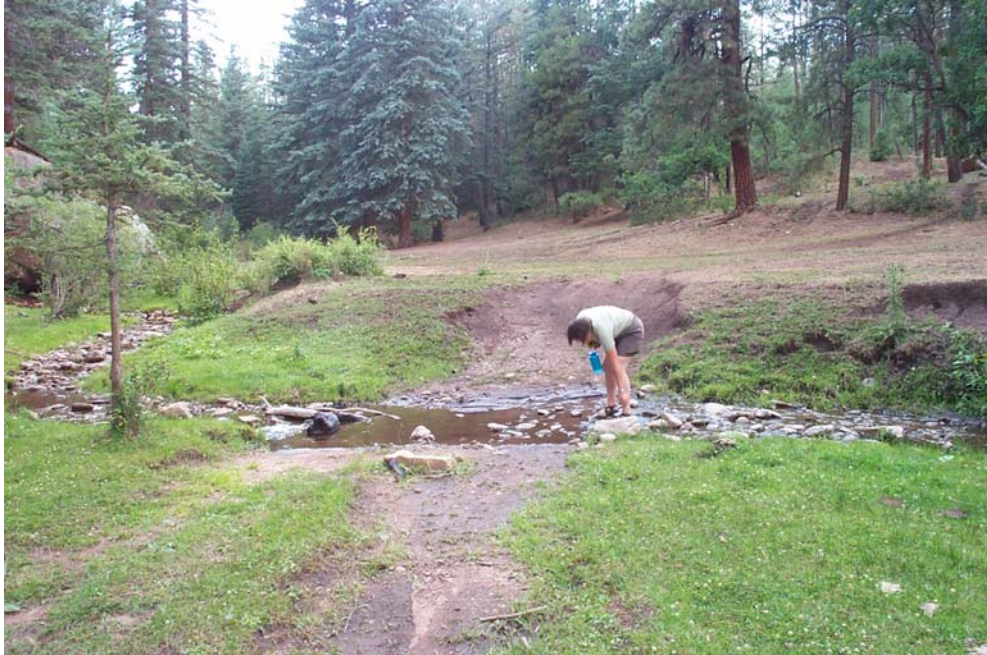
Photo 47. A user-created spur from FS Road 1161 increases the wetted width as well as erodes the banks increasing the already sediment-dominated substrate (17 July 2002).
