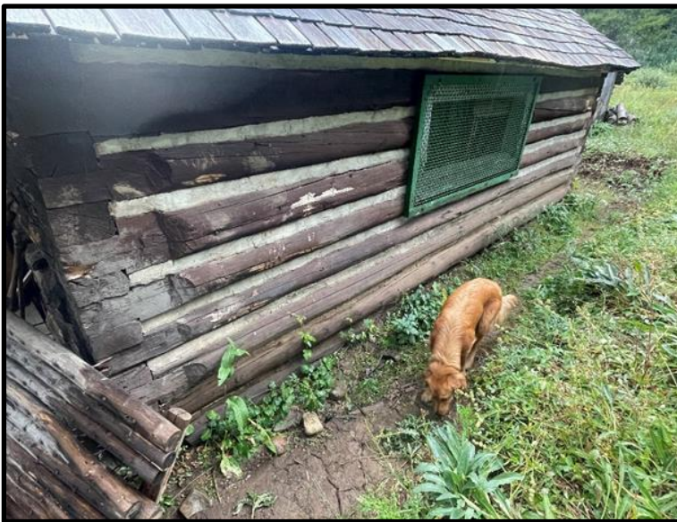
Sabado Cabin's North side. First sill log was completely rotten, second sill log had enough dry rot to require replacing.
