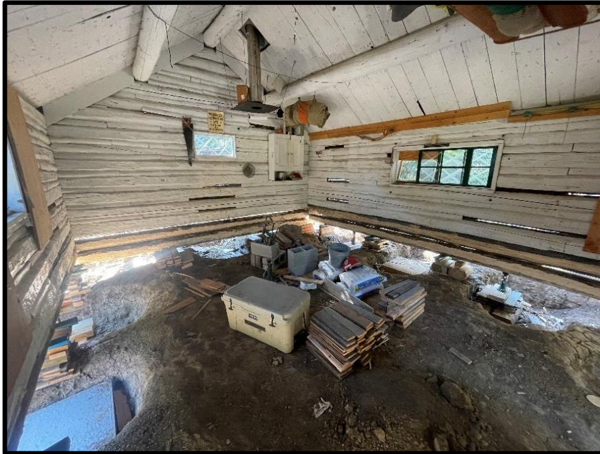
Interior picture depicting two logs replaced on each the north and west sides.
