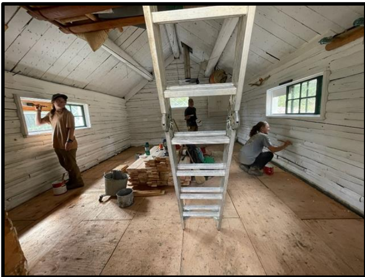
Schafer Meadows trail crew members paint the interior of the cabin before the flooring is installed.
