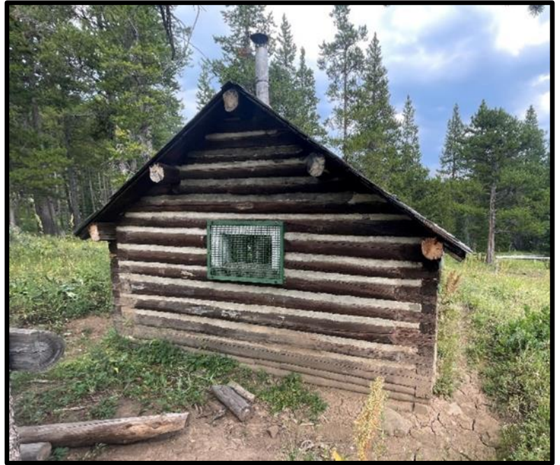
Sabado Cabin's West side. First spandrel log is completely underground, second spandrel log is half buried.
