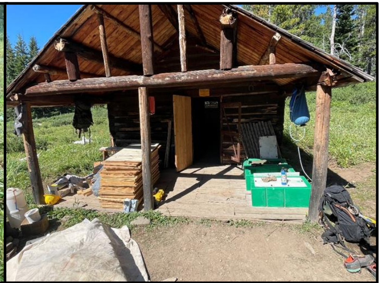
East side, showing porch floor completely below grade and rotten.
