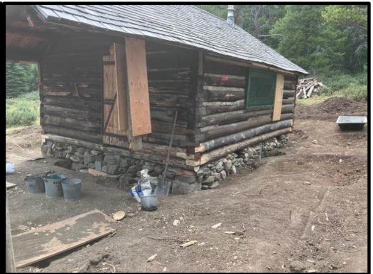
View from northeast showing replaced logs and rock foundation installation in process.
