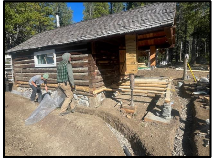
This picture shows the 1 st tier ditch, 2 nd tier French drain, and porch joists all under construction.
