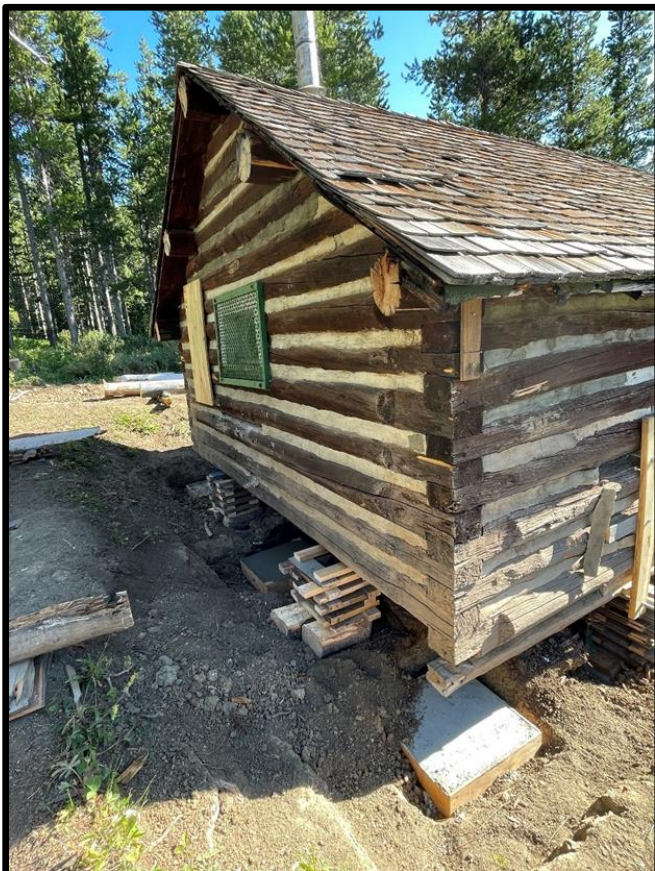
Two rotten spandrel logs removed from the west side of the cabin (left) and one rotten sill log removed from the south side (right). We would later determine there was enough rot in the second sill log on the south side to warrant complete replacement as well.
