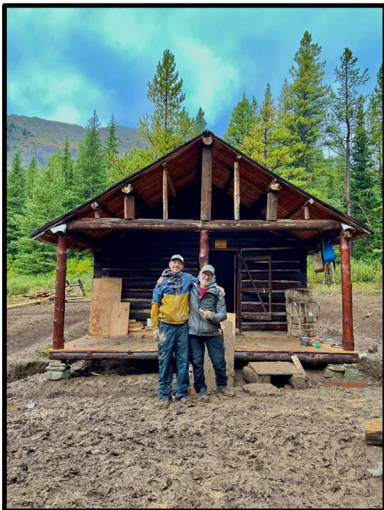
Caleb Fossee (left) & Carlos Florey (right) of Spotted Bear Ranger District pose in front of the finished project before hiking out on 8/31/2023.
