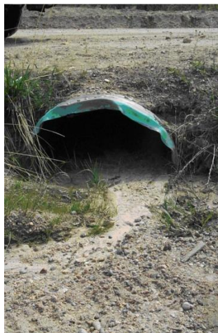
Photo L. Steel 18" culvert inlet, 20-80% occluded by sediment. Note that there is some crushing, but this is not significant because it does not cause any problems, and occlusion is the main issue here.
