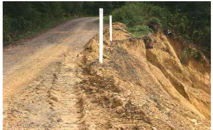
Photo AA. Road related landslide. This fill failure initiated at the point where a culvert discharges to the hillslope.
