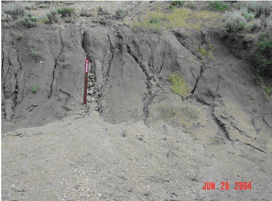
Photo G. Badly rilled cut slope following high intensity rainfall event.
