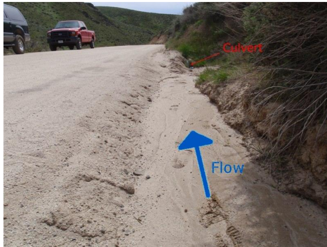
Figure 9. A sediment pile below a ditch relief culvert.
