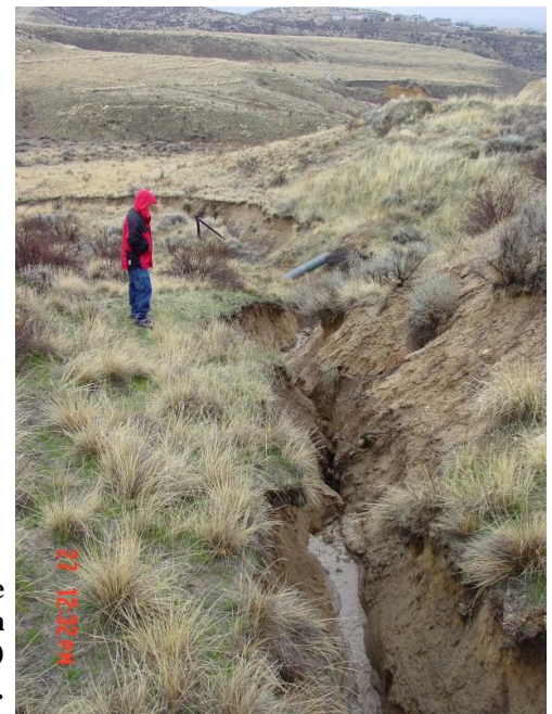
Photo Y. Active gully below culvert due to excessive contributing road length. Note the V-shaped cross section and steep side slopes. This active feature continues over 700 feet to the main valley bottom.
