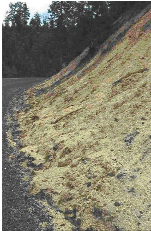
Photo E. A severely raveling cutslope in granitic saprolite. The ditch has been obscured by the accumulated apron of debris
