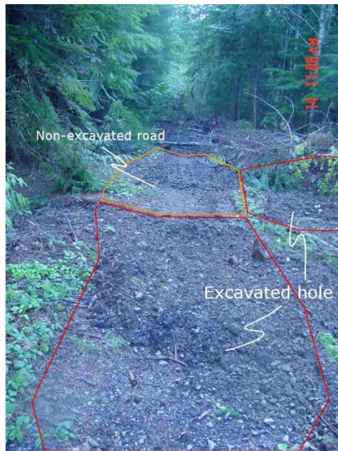
Photo D. Decom potholed road.
