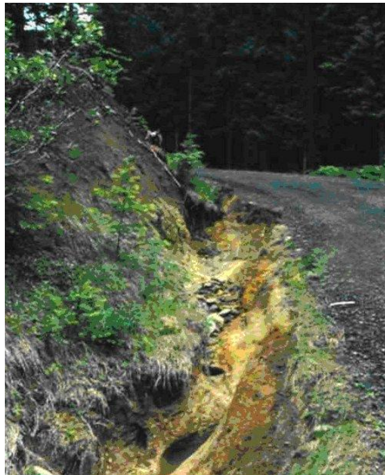
Photo H. Badly gullied ditch after large runoff event
