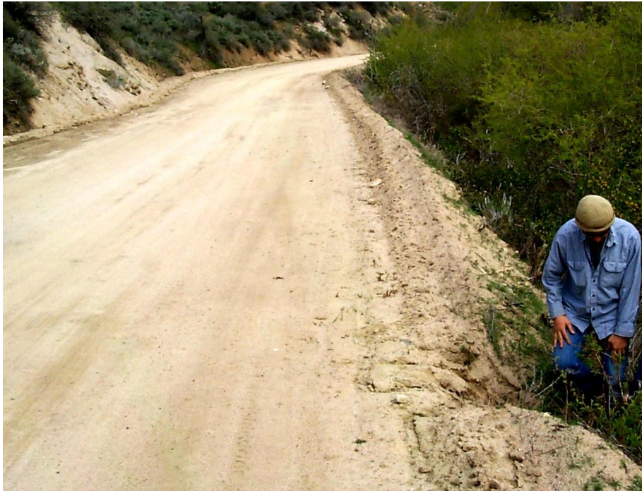
Photo Q. A non-engineered drainage at a broken berm. Water flowing along an outside berm is diverted over the fillslope. The fill erosion in this case would meet the 5 cubic foot minimum.
