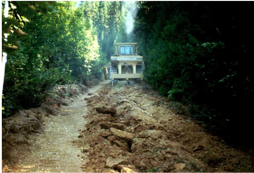
Photo B. Ripped road.
