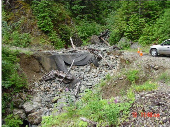
Photo S. A washed out stream crossing.
