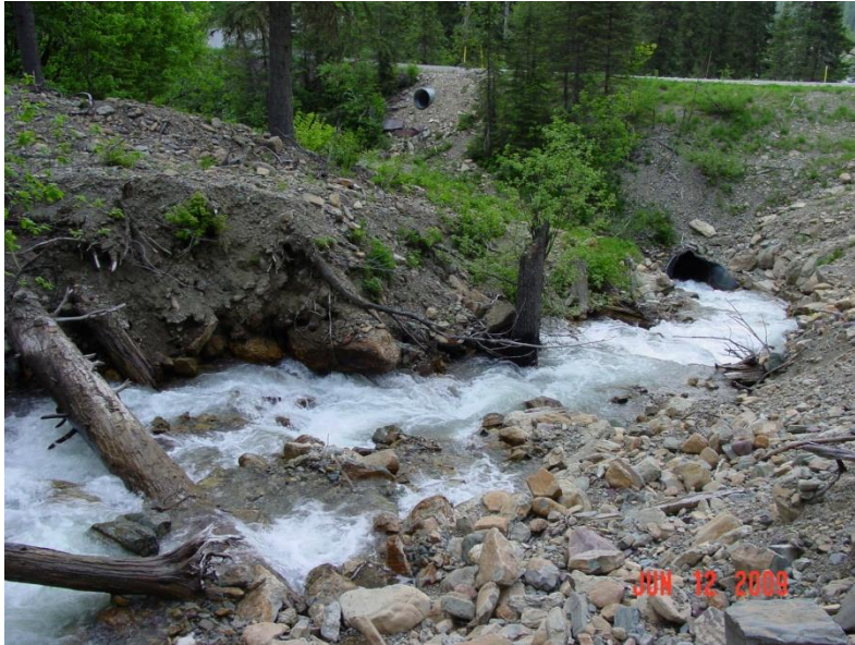
Photo T. Debris flow at a stream crossing. Notice the mass of sediment intermingled with buried logs.
