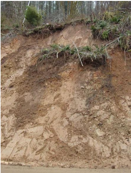
Photo F. A slumping cutslope.
