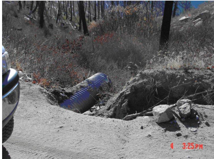
Photo I. Fill erosion caused by flow around culvert pipe.
