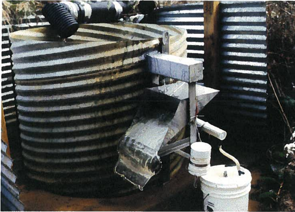
Figure 13. Tipping bucket and flow splitter in operation. The 20 gpm (66 lpm) design is shown.
