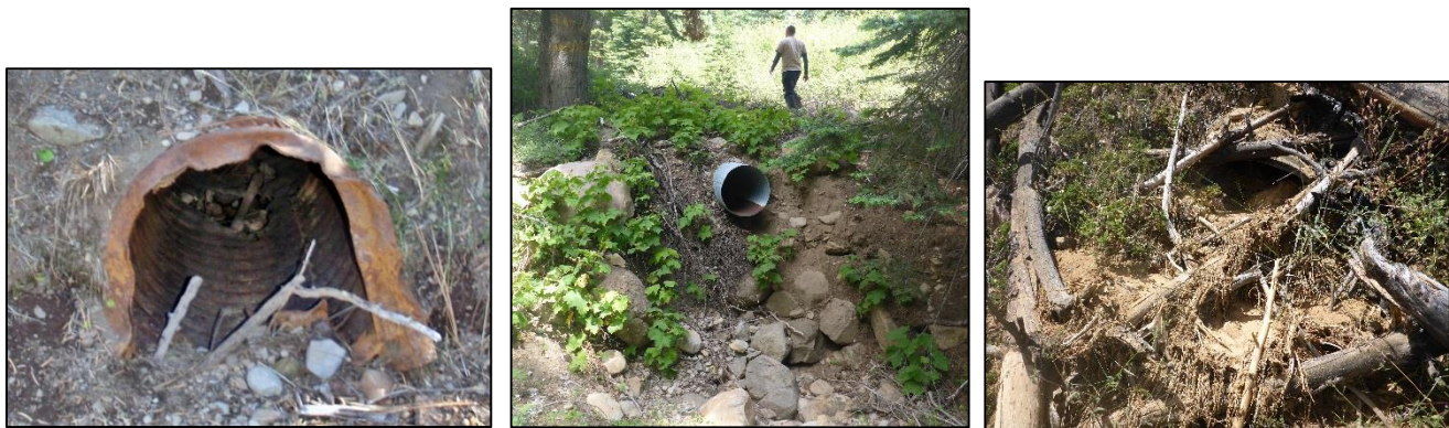
Figure 40. Problems with ditch relief culverts. The left culvert is rusted through. The middle culvert is set high in the fill. The right culvert has an occluded inlet.
