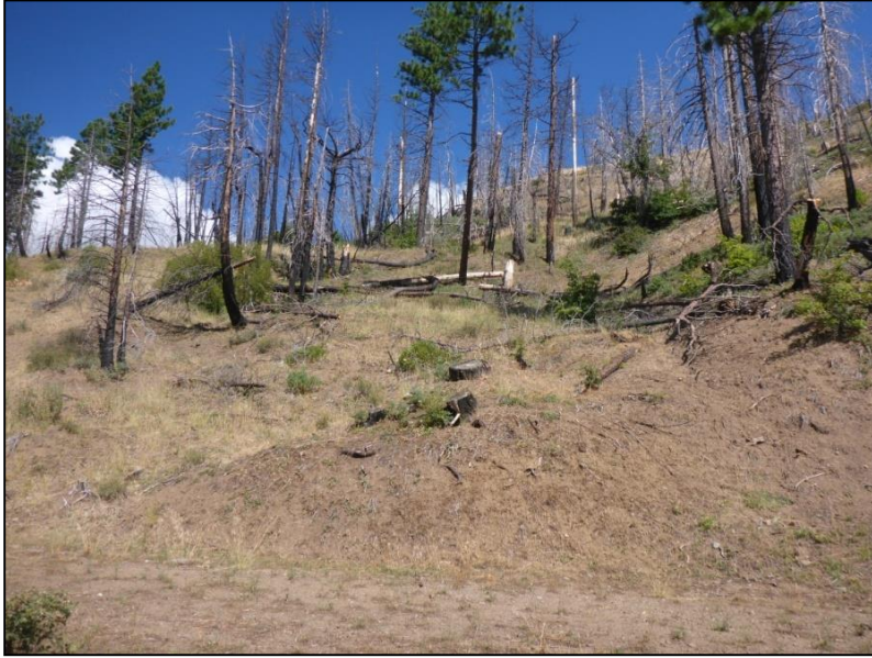
Figure 21. Cutslope failure type landslide.
