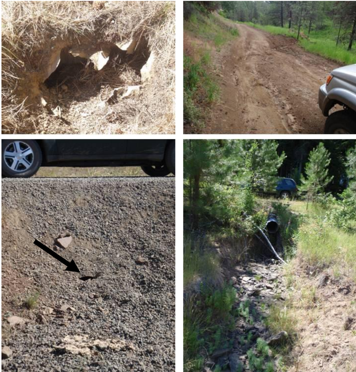
Figure 15. Examples of drain point condition problems, clockwise from upper left: crushed and occluded ditch relief culvert (road 2200 near Turner Mountain), eroded waterbar (road 2200-027), buried ditch relief culvert (road 2128 near Wilson Prairie), and ditch relief emptying into gully below road crossing (road 2519).
