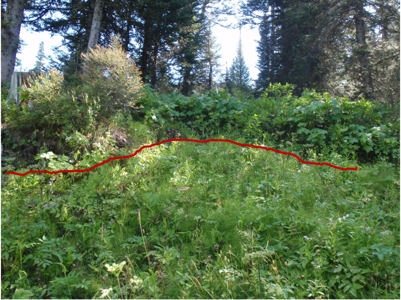
Figure 6. Slump in cutslope near the end of the upper 046 spur road. Red line indicates approximate scarp base.
