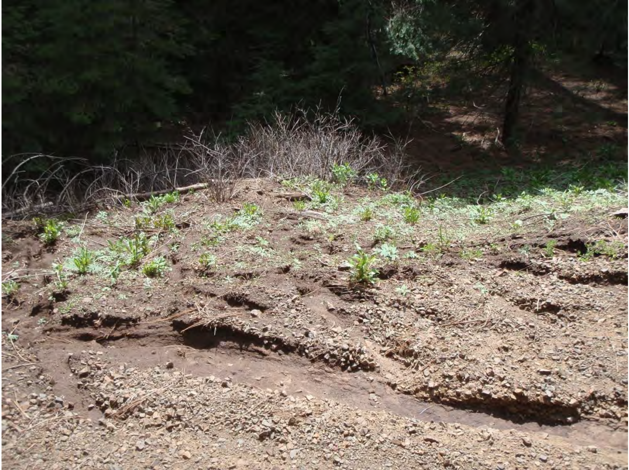
Figure 10: Gully and rills along control road. These extend from the road surface across the fill and onto the hillslope below.
