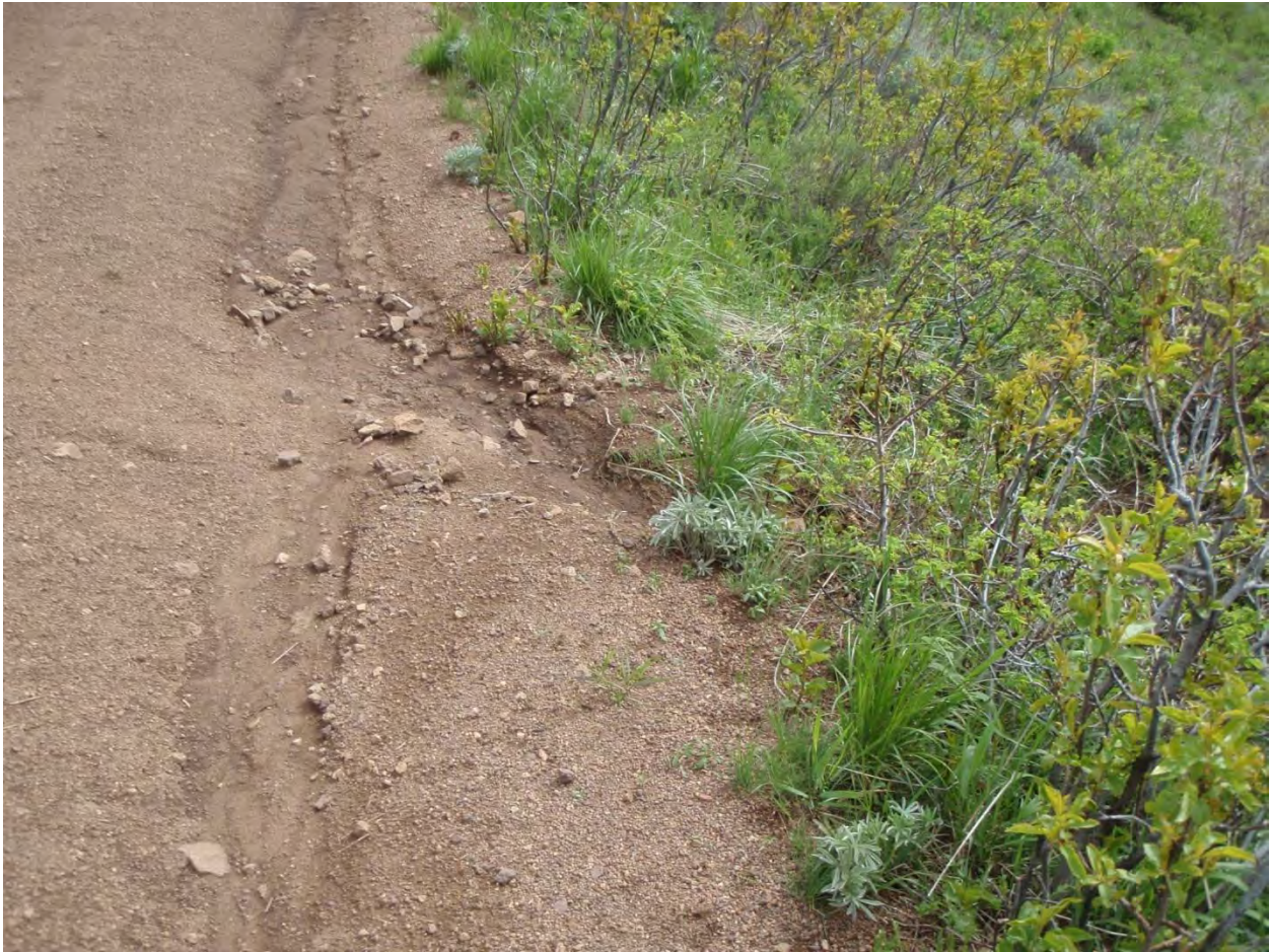
Figure 9: Non-engineered drain formed along control road.
