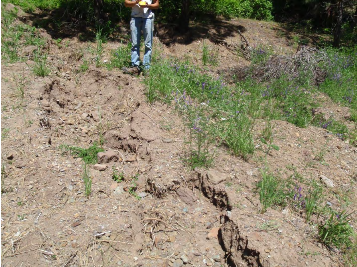
Figure 6: Gully crossing recontoured road.
