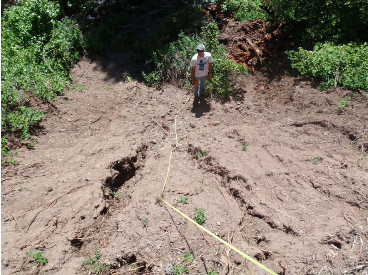
Figure 7: Slump in recontoured fill. View is from top of scarp.
