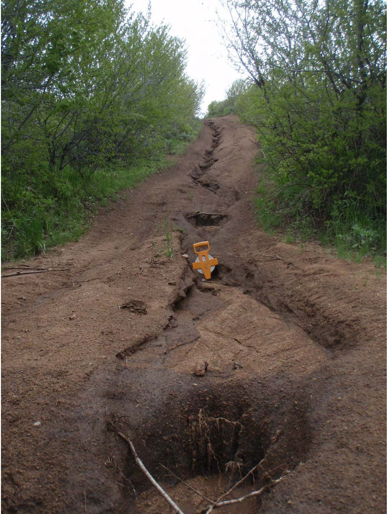
Figure 8: Gullied flowpath on control road 500100500.
