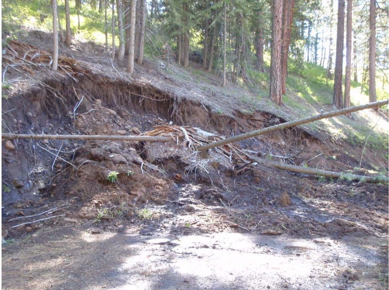
Figure 11: Cutslope failure along control road 50029/50473/50007?.
