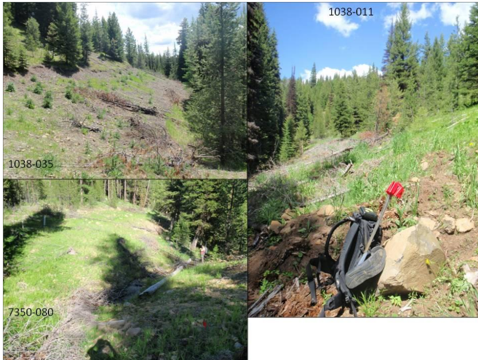
Figure 10: Typical road conditions during the post-storm inventory. The section of the 1038-011 shown here (right) was connected to the stream during treatment.
