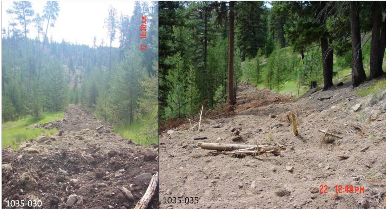
Figure 8: Post-treatment road conditions. Ripped / tilled road on left; recontoured road on right.
