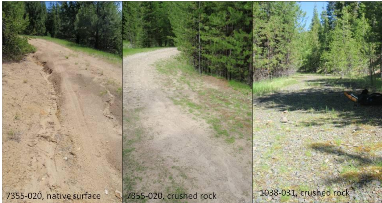
Figure 14: Typical control road conditions, post-storm.
