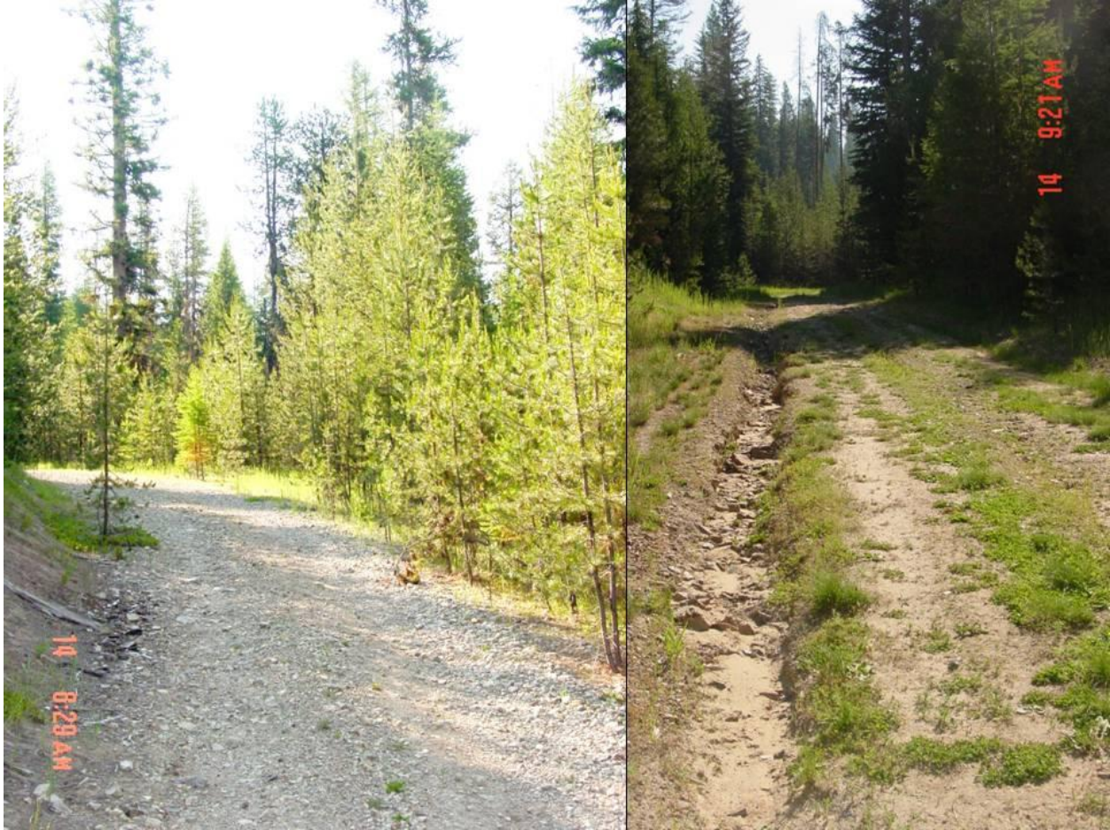
Figure 12: Typical control road sections, pre-storm. Crushed rock surface on left; native surface with gullied wheel track on right. Both pictures from the 7355-020 road.
