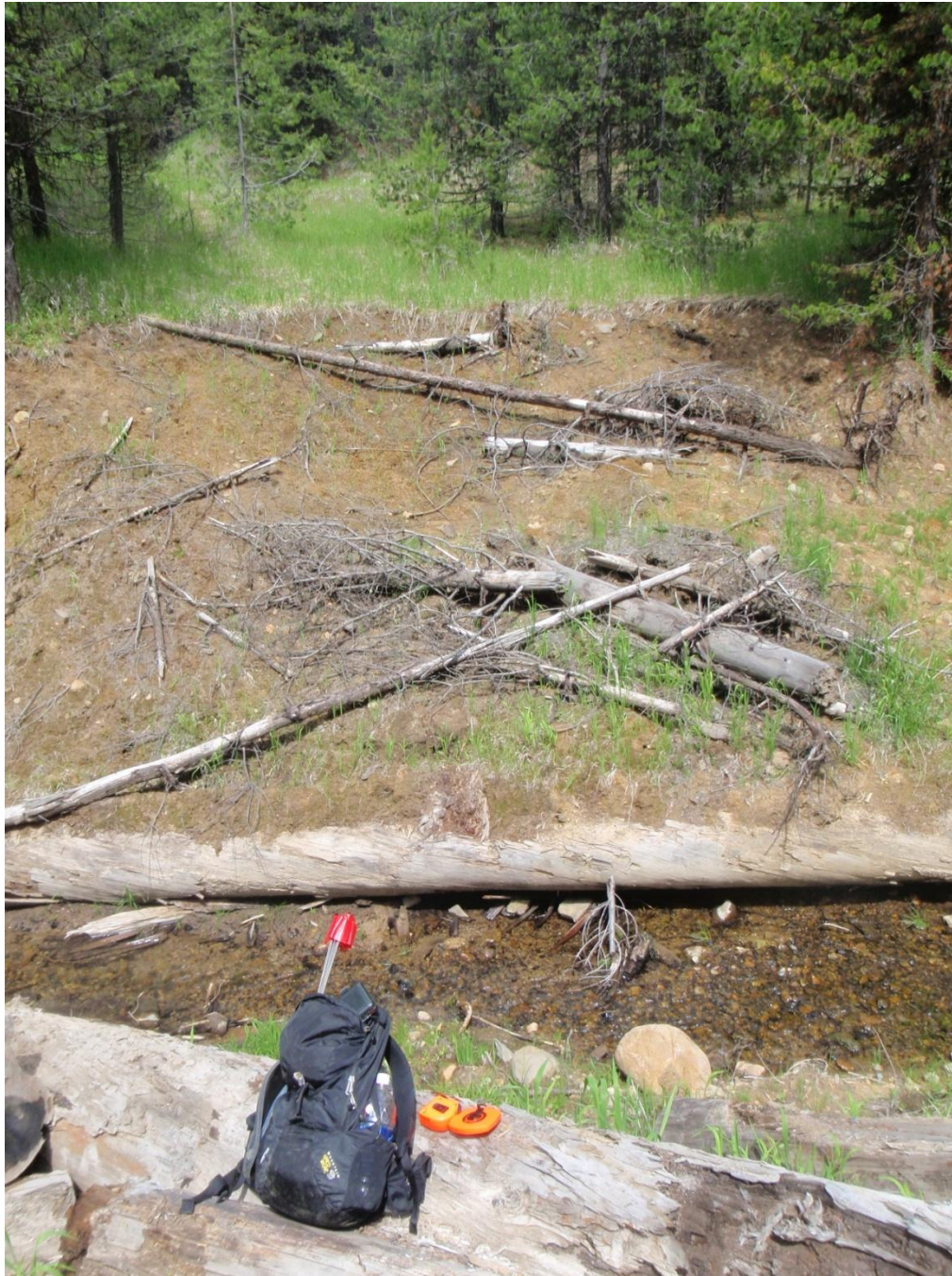
Figure 23: Excavated stream crossing with log placed to prevent erosion. The field crew recorded a landslide in the sideslope of the excavation at this location.
