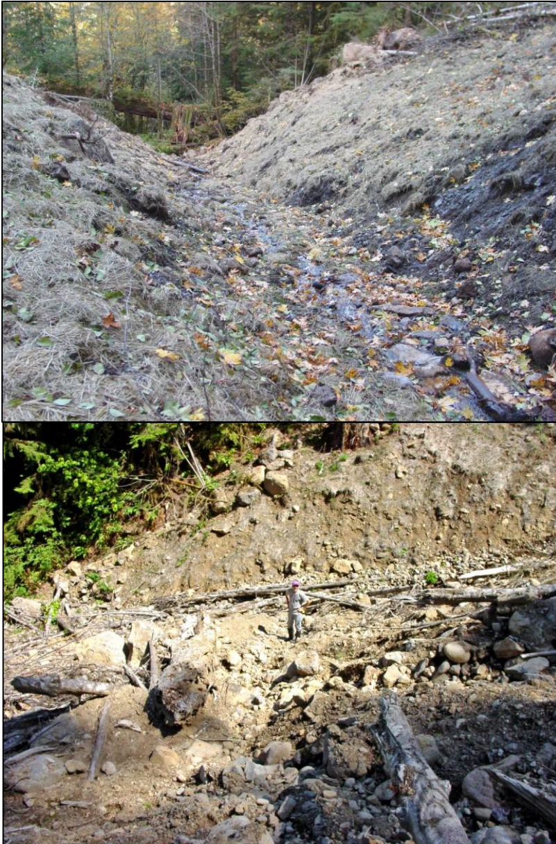
Figure 10. Excavated stream crossing on NFSR 1211000. Condition before storm (top) and after storm (bottom). 121 yd 3 of sediment was eroded from this crossing by the storm.
