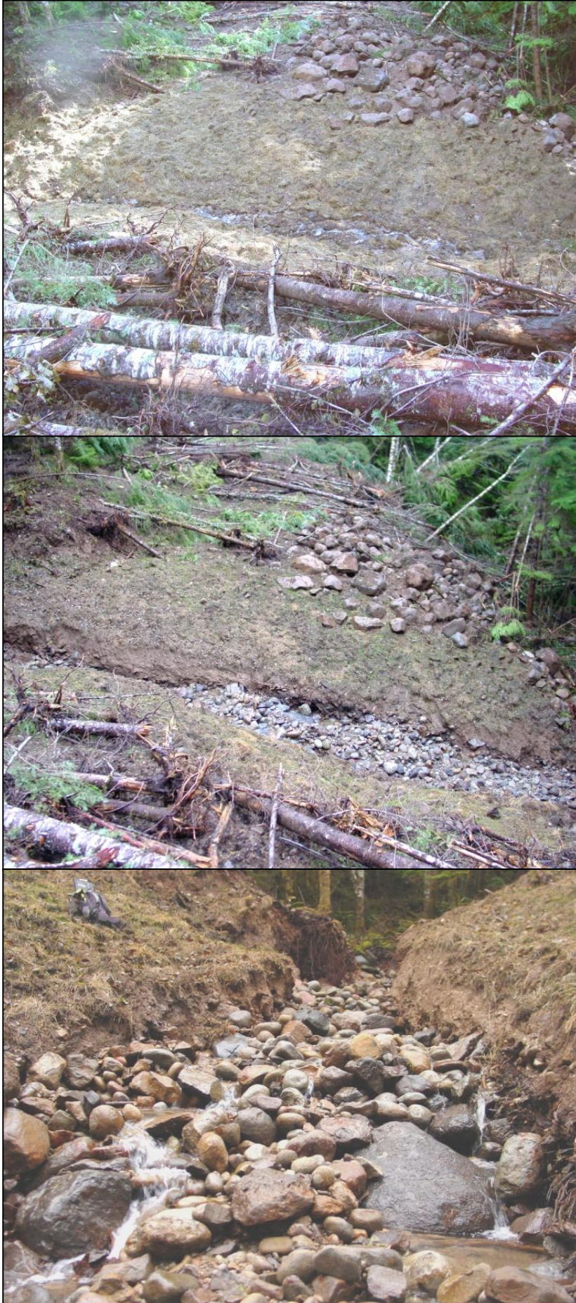
Figure 9. Excavated stream crossing on NFSR 1210428. Condition before the storm (top), with some scour already present; view from same location after the storm (middle); and view in the channel after the storm (bottom). 178 yd 3 of sediment was eroded from this crossing during the storm. This crossing was located on an unstable stream channel that runs through an historic landslide (T. Parker, personal communication, 2011)
