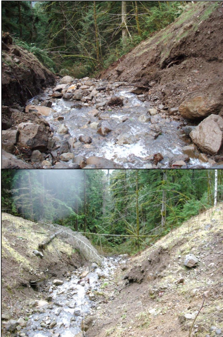
Figure 15. Stream crossing in road 1211 in 2008 after the initial 25 year recurrence interval storm (top) and in 2012 after the more recent 25 year recurrence interval storms (bottom). There may be some side slope erosion, but no new major erosion was observed.
