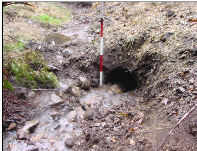
Figure 12. Second pipe that was left in after the crossing excavation and was flowing water at the time of the survey.
