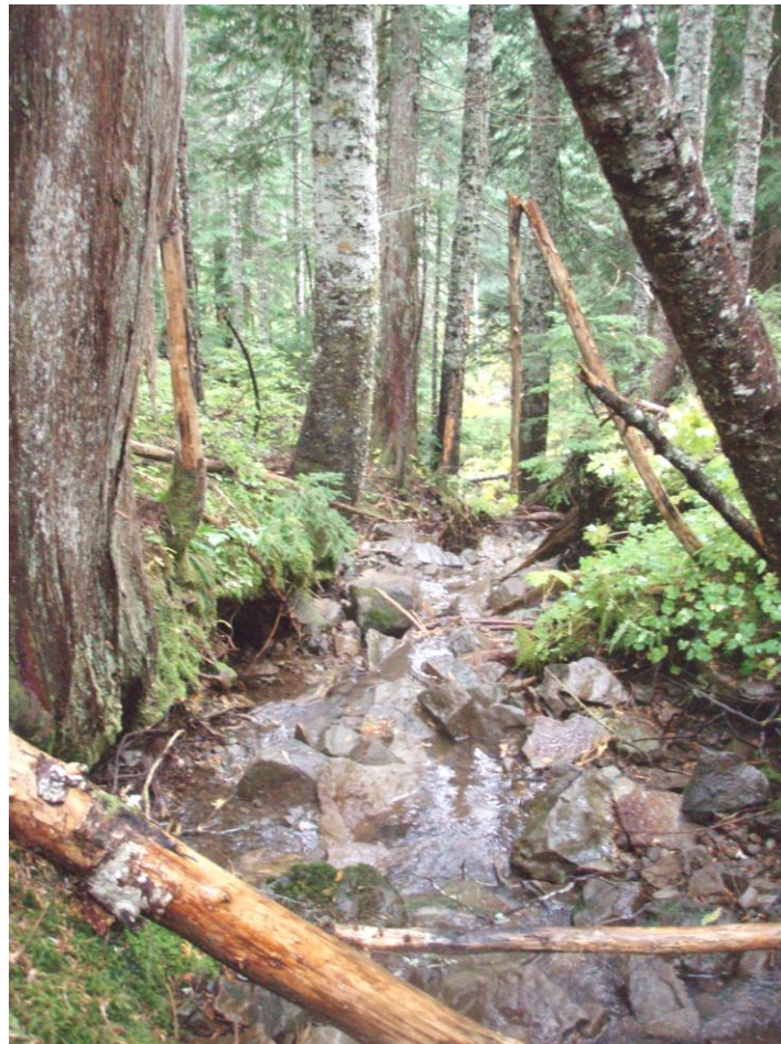
Figure 13. Stream diversion of the Little Sandy River on the 1200-222 control road. This was present during the pre-storm survey.
