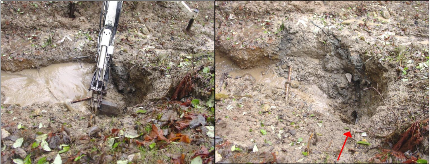
Figure 11. Excavated crossing on NFSR 1211000 that had a second buried pipe. The spider excavator dug down to the pipe opening (top), and exposed the inlet (bottom, with arrow) before it was pinched closed and re-buried.
