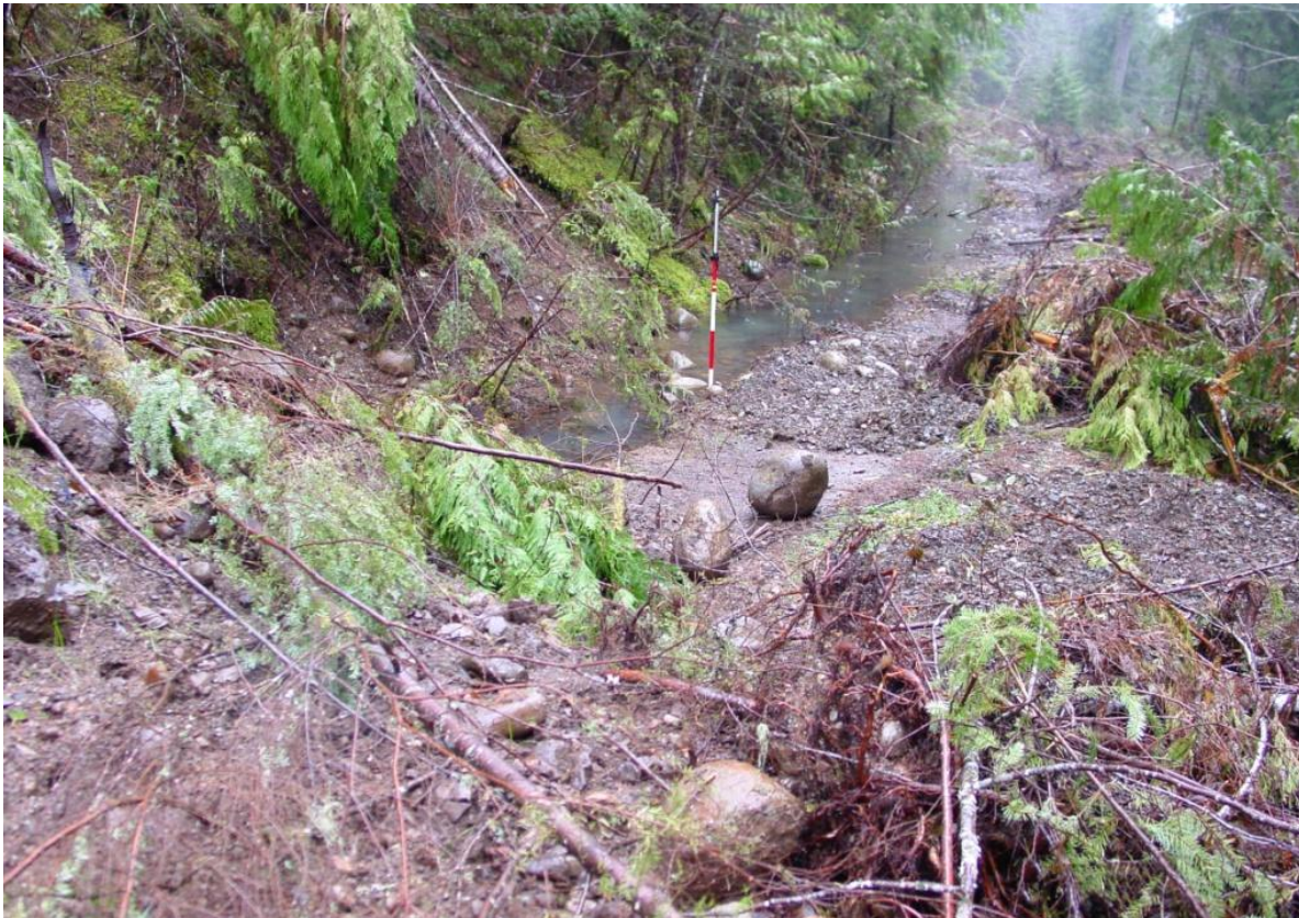
Figure 16. Pool behind a fill pile from a stream excavation on NFSR 1210428 that was placed on the uphill side of the crossing, preventing the water running down the ditch from draining.
