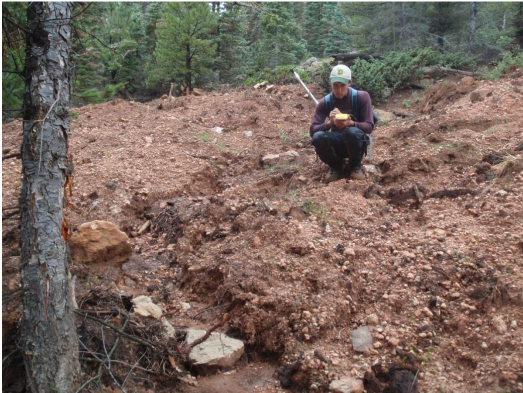
Figure 6: Hillslope gully crossing recontoured road.
