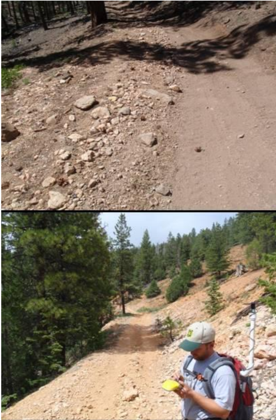
Figure 9: Typical pre-treatment road conditions.
