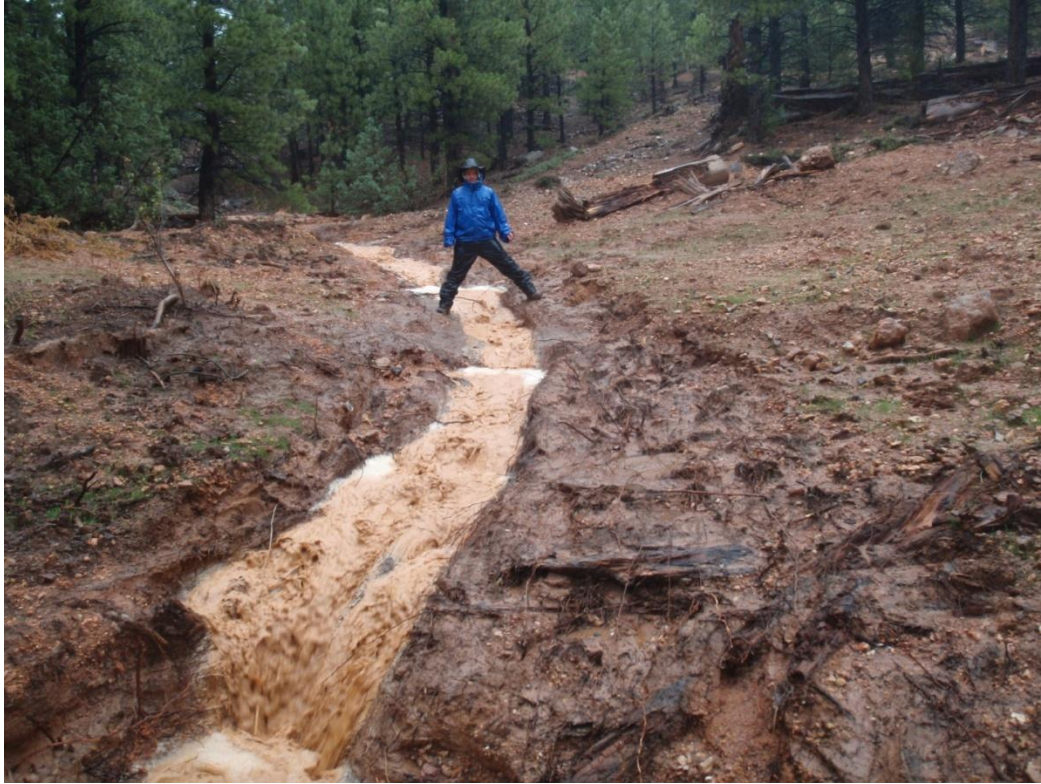
Figure 5: Erosion at intermittent stream crossing, erosion extent is wider than Scott's height. Pictured flood flow generated by 0.20" of rain in 30 minutes.
