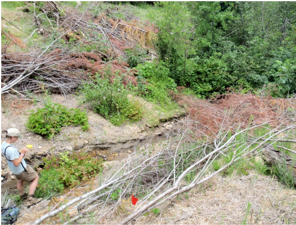
Figure 10. Excavated stream crossing on road 5105 (Yakus). Note the channel incision and living vegetation on the side slopes. This represents a “typical” excavated stream crossing for these roads.
