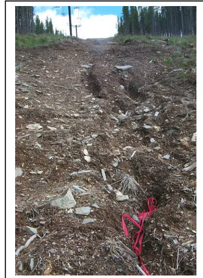
Fig. 35. 2005-erosion above road
