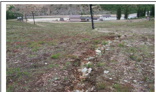
Fig. 43. 2005-headcut above lodge on Gold Run
