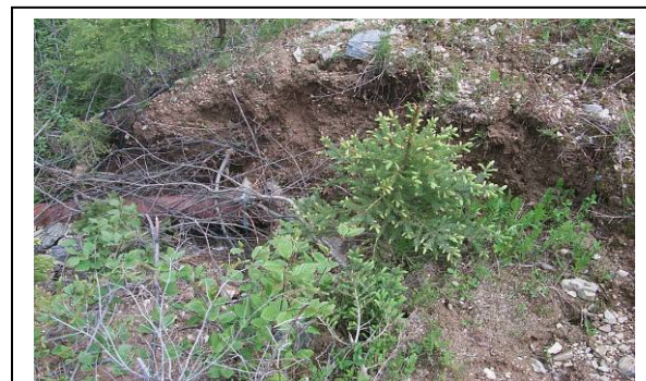
Fig. 47. 2005-broken culvert below lower lift
