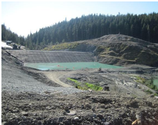
Photo from North end of Lower Slate Lake looking South towards Tailings Disposal Facility. 09/16/2010.
