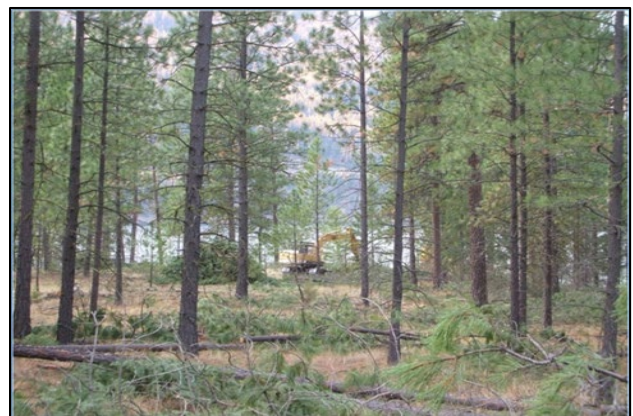
Figure 4. Thinning treatments to reduce tree density and prevent insect-caused damage that were supported with FHP management funding and technical expertise.
